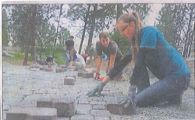
Coeur d'Alene Bible Church volunteers Grace Moehling and Clay Finney install pavers at the new amphitheater/outdoor classroom next to the Harbor Center and the Centennial Trail in Coeur d'Alene last Sunday. The new space will be used for education and recreation and is open for student and community use. More features will be added in the coming weeks and months.
