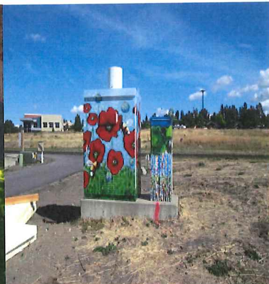
Bellerive Monitoring Station Discharges to Spokane River
